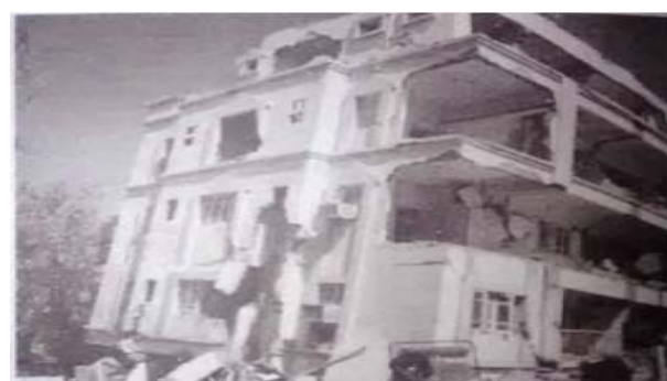
Fig. 5: Failure of the reinforced concrete building
