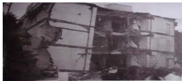
Fig. 4: Failure of reinforced concrete columns with floating columns
