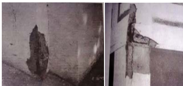
Fig. 7: Damage due to corrosion of steel at column force and at beam column joint
